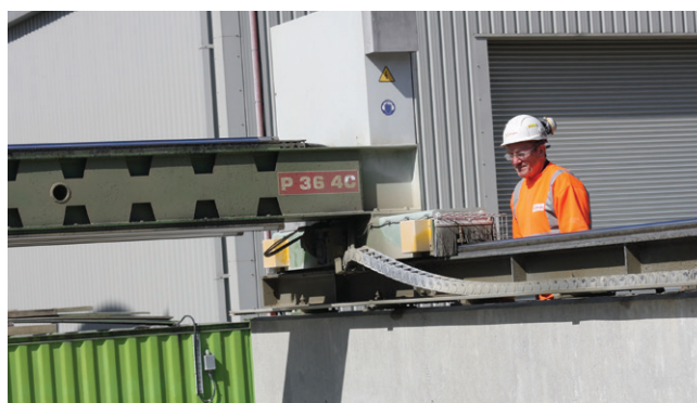
Fig 2b: Operator position on mezzanine
