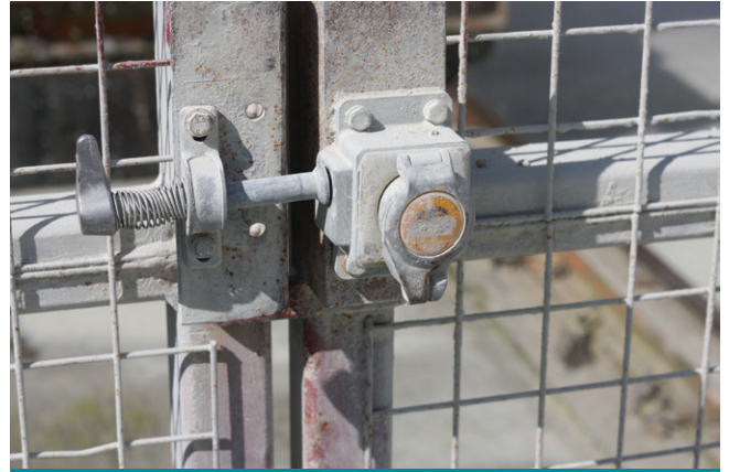
Fig 5d: Perimeter guarding and interlocking
